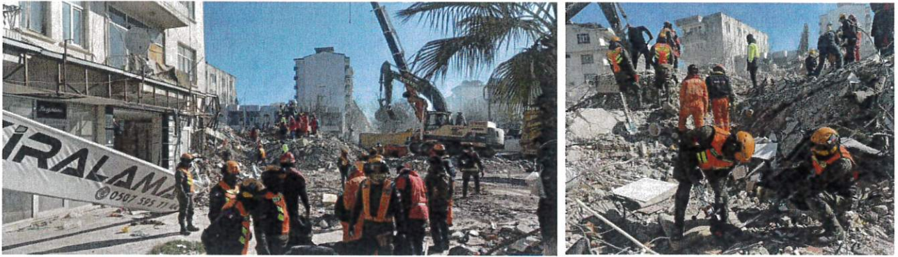
On 13 February 2023, Philippine USAR team geared up for SAR Operations on a collapsed apartment complex believed to house 100 persons.
