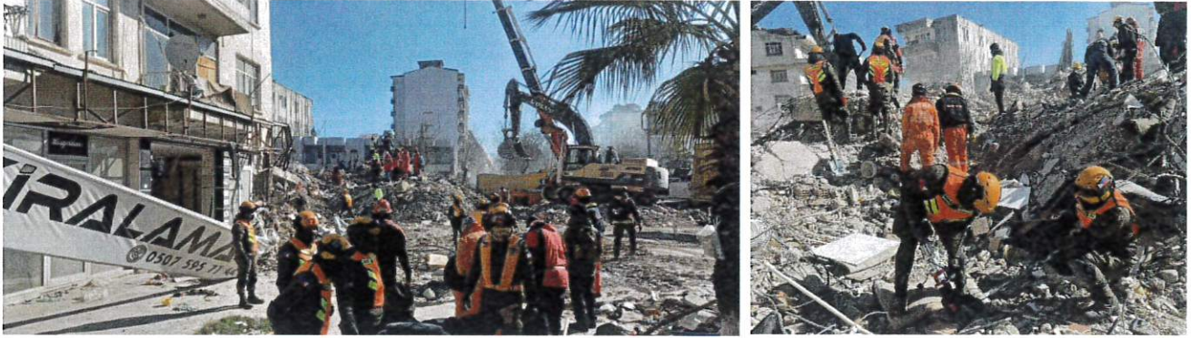
On 13 February 2023, Philippine USAR team geared up for SAR Operations on a collapsed apartment complex believed to house 100 persons.
